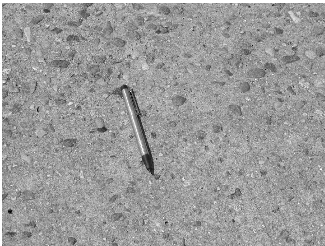
Figure 7: Exposed aggregate in the wheel path on the Ryå Bridge after 20 years exposure. In the bottom of the picture, the original brushed surface texture can be seen
