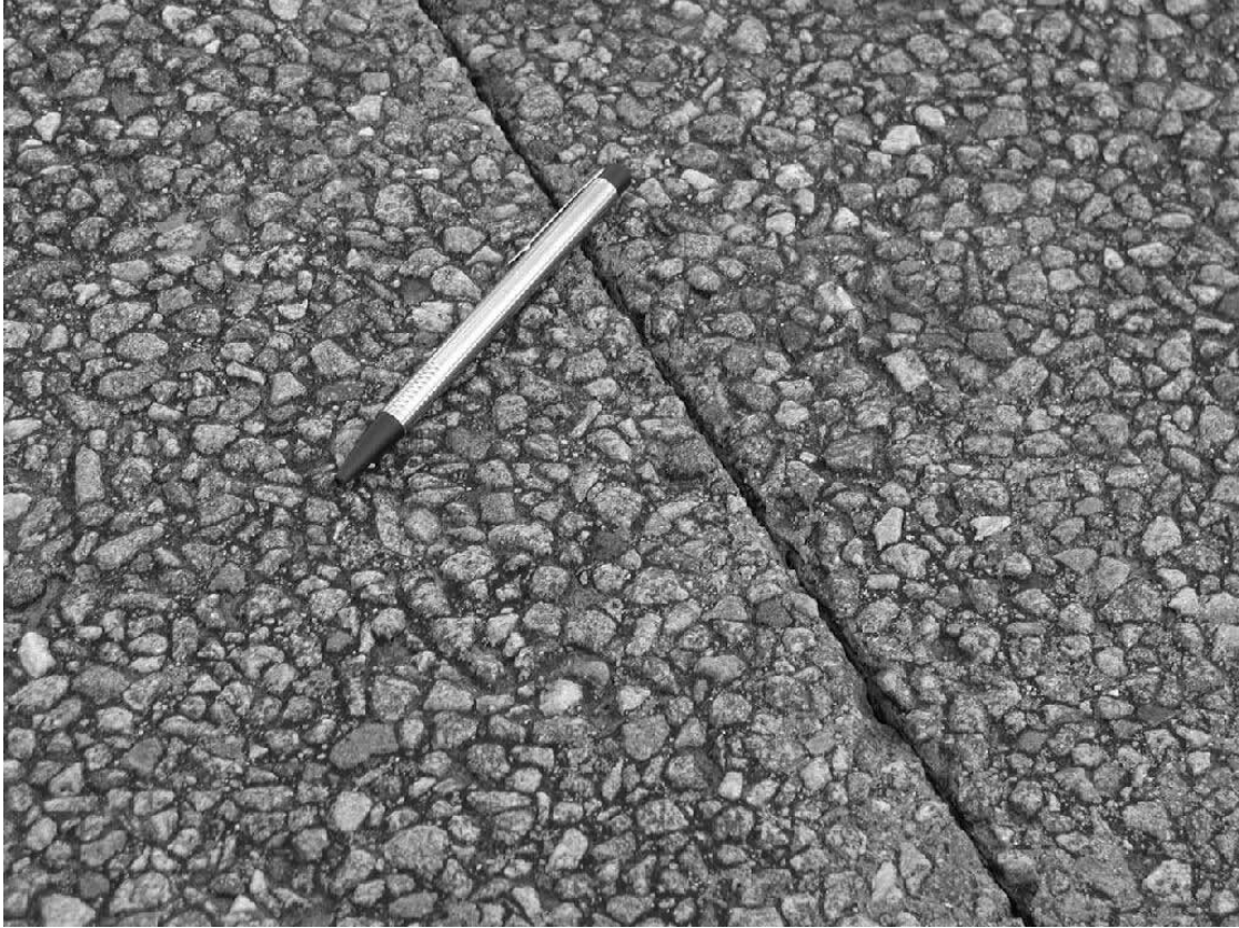
Figure 23: Surface and a transverse sawn crack of the ECOPAVE road after 6 years of service.
