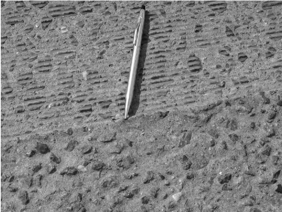
Figure 17: Surface of the Slagslunde Road. In the bottom of the picture the original exposed surface, in the top the bump-cutted surface. Photograph taken in October 2001
