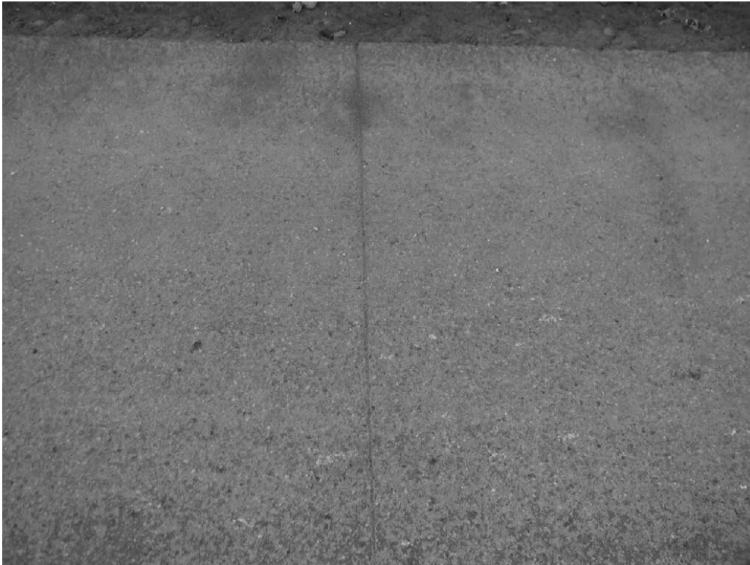
Figure 20: Surface of the road. No damage at the sawn joint or the edge can be seen.
