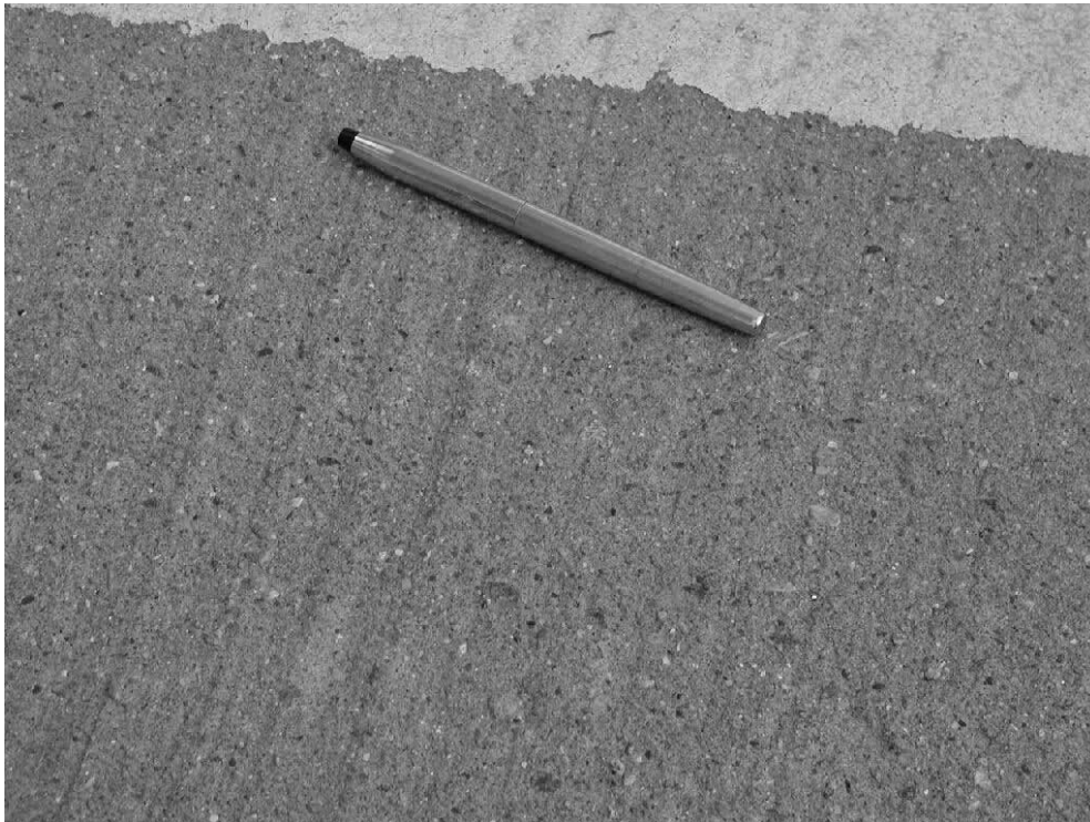
Figure 13: Surface of Bredal Bridge after 15 years exposure
