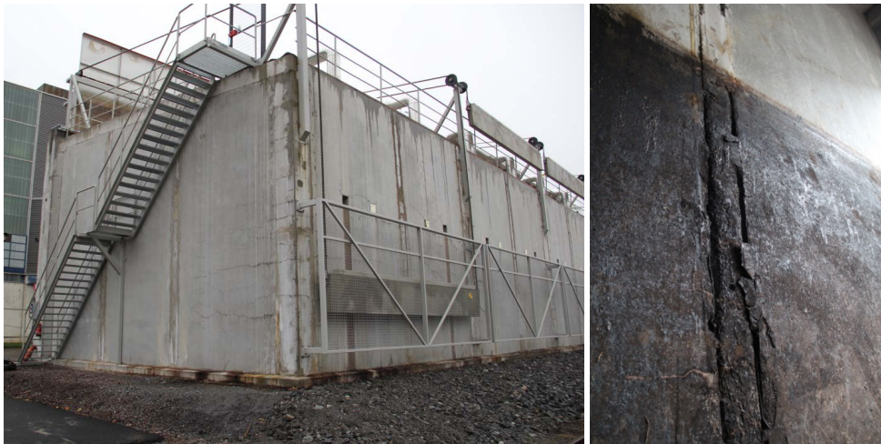
Figure 1 – Left: Outside cracking can be detected both in precast concrete panels and in casted joints. Right: Cracking and spalling in casted joint inside of the chamber. Photo area is app. 2.2 x 3.3 m 2 .
